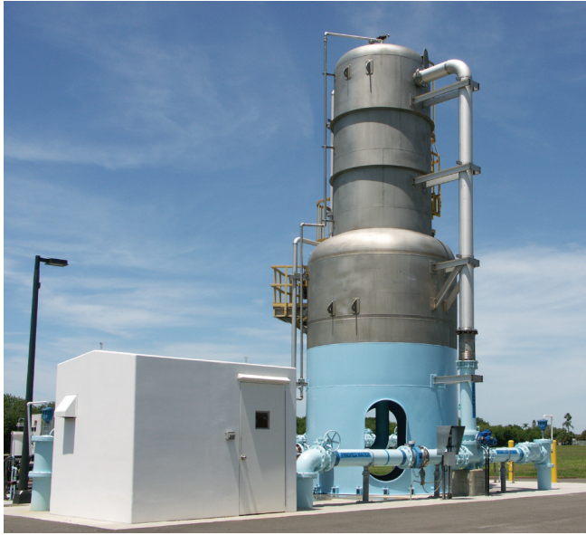
Single Stage Stainless Steel Vacuum Degasifier with integral clear-well storage compartment on an ASR (Aquifer Storage Recovery) project – Florida
